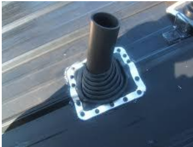
Figure 4 – A rubber boot is shown on a roof vent pipe fastened to the metal roof with sealant and small sheet metal screws.
