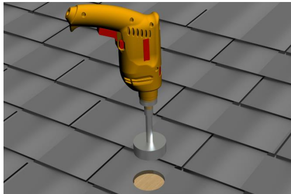
Step 2: Use a 3 inch hole saw to make a clean hole in the metal roof shingle.
